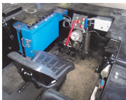
Q800 Drive installed
